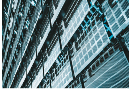
Wall of solar panels
